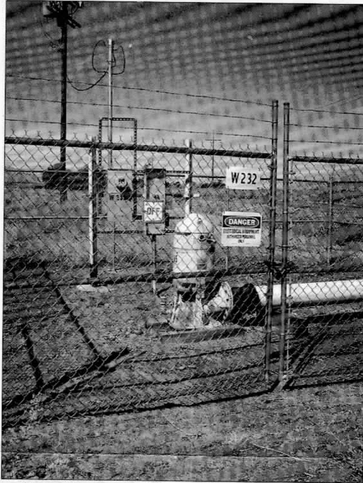
Los Angeles Department of Water and Power Well 232, south of Big Pine, is currently in "off" status. The Inyo County Water Department is looking at ways to improve or adjust the current "on/off" protocols that govern pumping in the Owens Valley. Photo by Jon Klusmire
