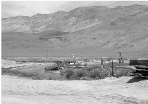
Work proceeds on the Lower Owens River Project near the aqueduct intake.
